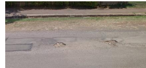
POTHOLES IN RIVERTON ROAD
